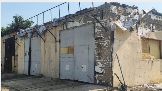
Photo of the fire station damaged following attacks in Stepnohirsk on June 2, 2025. Source: State Emergency Service in Zaporizhzhia Oblast. 129
